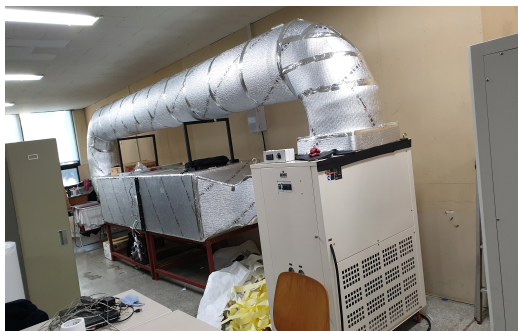
The actual use of heat pump equipment
